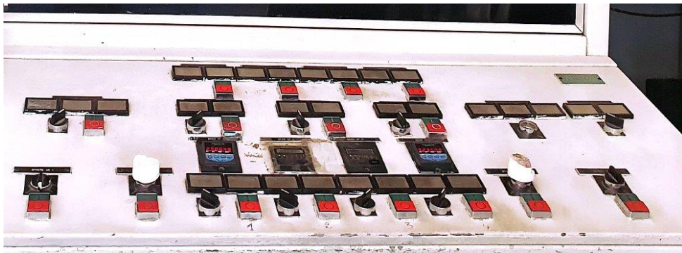
Figure III- 11 : Console de supervision
